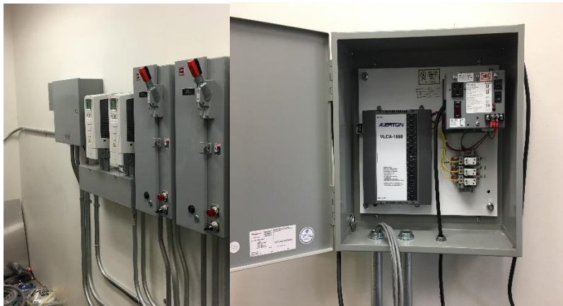
Figure 22. The Allerton control module and installation images
