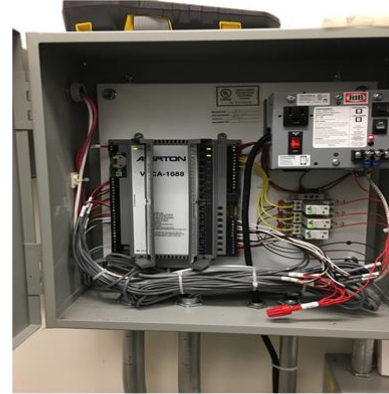
Allerton BMS controller
