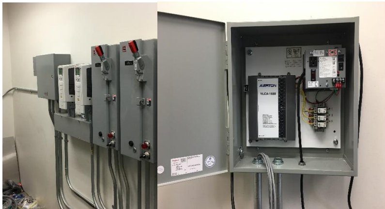
Figure 22. The Allerton control module and installation images
