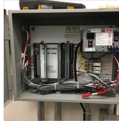
Allerton BMS controller
